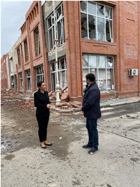
Destroyed shopping center-Photo 6.
